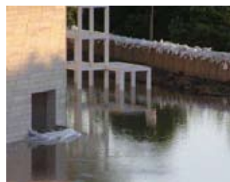
North side of IATL after 21-24 inches of water invaded the building. (Photo by Mark Arnold)
